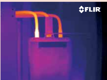
Bad connection in a cable.
