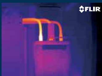
Poor connection and internal damage
